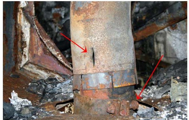
Poor maintenance failed to properly tighten engine pipe exhaust clamp was the cause
