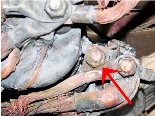
Improperly factory installed battery cable on the solenoid caused five new vehicles to burn.
