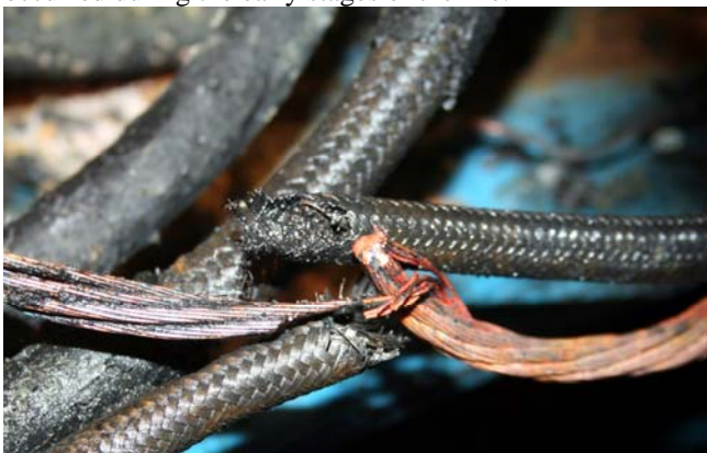
Poorly secured battery cable and fuel lines eventually wore through causing short circuit and fire
