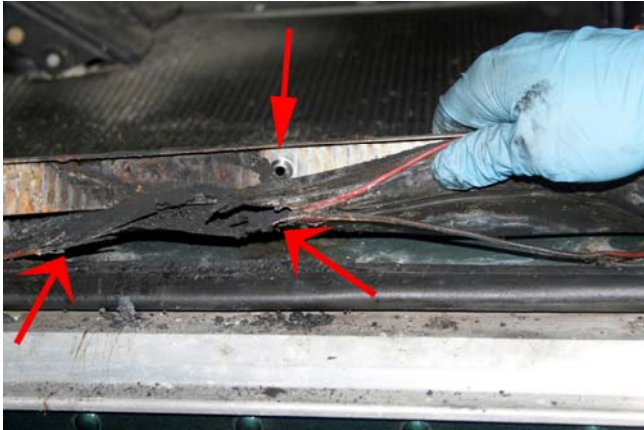
Wire were installed under metal trim and hold-down screw penetrated wire insulation causing short to ground
